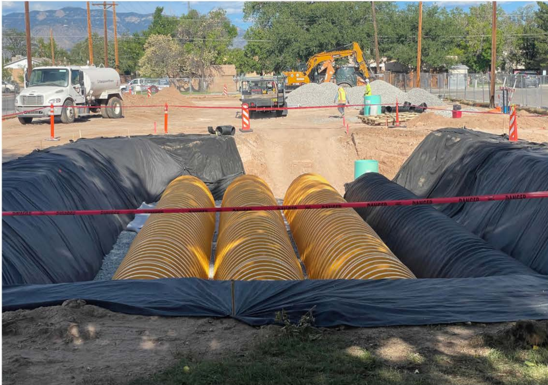
A NEWLY INSTALLED RAINWATER INFILTRATION SYSTEM UNDER THE PARKING LOT OF THE REDESIGNED CRISIS TRIAGE CENTER AT UNM HEALTH SCIENCES.
